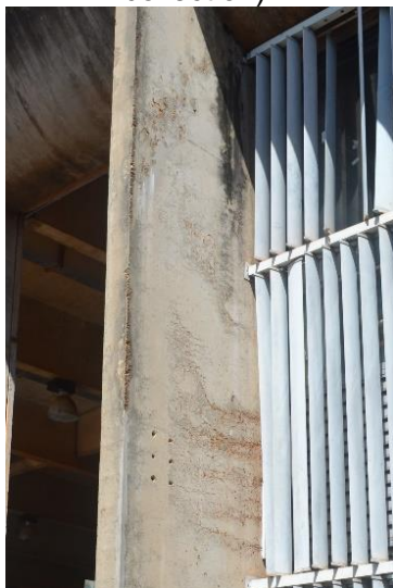
Figure 42: segregation due to manufacture flaws on Pillar 474 (private collection)
