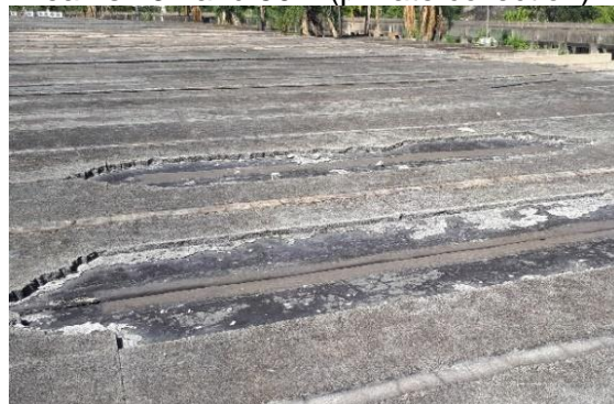
Figure 58: Removed mechanical protection and waterproofing between Beams 492 and 501 (private collection)
