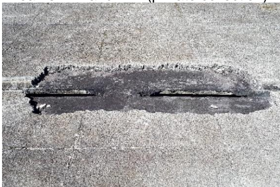
Figure 57: Removed mechanical protection and waterproofing between Beams 471 and 474 (private collection)
