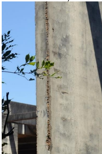
Figure 52: segregation due to manufacture flaws on Pillar 504 (private collection)
