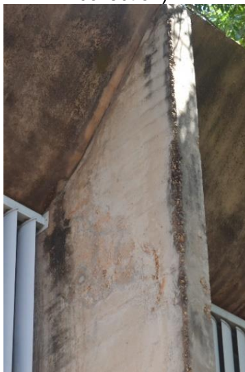
Figure 43: segregation due to manufacture flaws on Pillar 539 (private collection)
