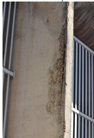
Figure 44: segregation due to manufacture flaws on Pillar 561 (private collection)
