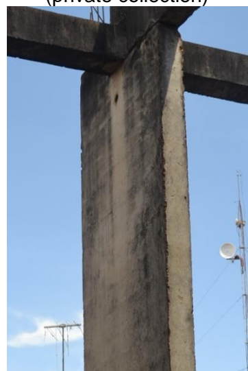
Figure 56: stains due to humidity on Pillar 570 (private collection)
