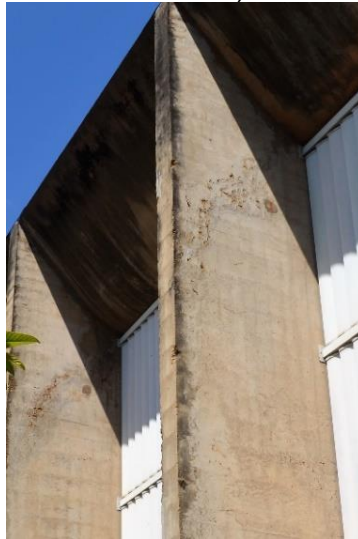
Figure 49: Efflorescence on Pillar 501 (Private collection)
