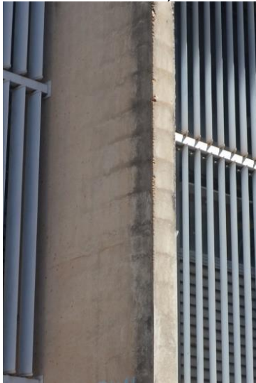
Figure 48: Efflorescence on Pillar 480 (Private collection)
