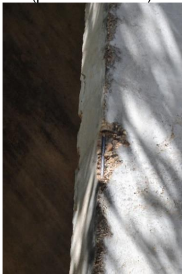
Figure 46: reinforcement corrosion on Pillar 552 (private collection)
