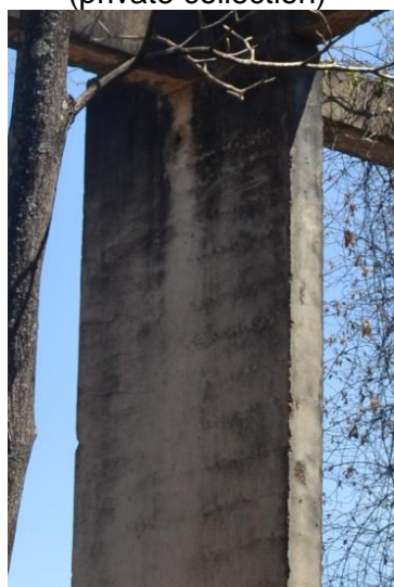
Figure 54: stains due to humidity on Pillar 477 (private collection)
