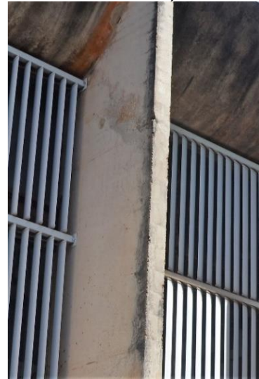
Figure 50: Efflorescence on Pillar 576 (Private collection)
