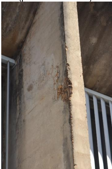
Figure 45: reinforcement corrosion on Pillar 483 (private collection)
