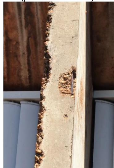
Figure 47: reinforcement corrosion on Pillar 570 (private collection)
