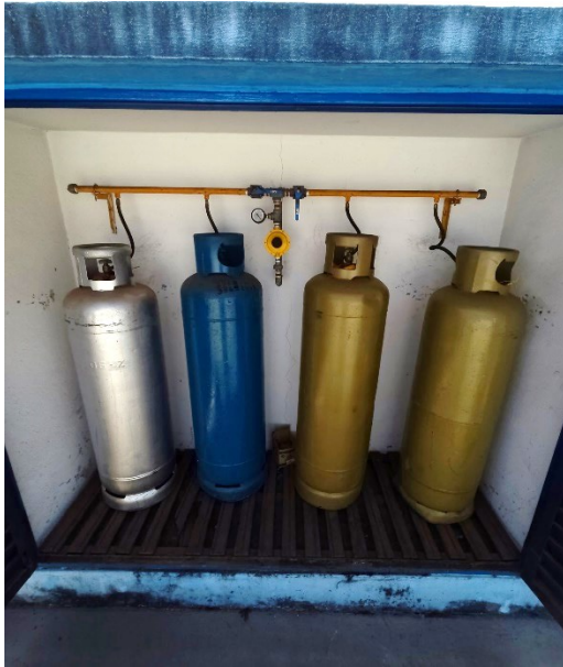
Figura 106 – Central de GLP.
