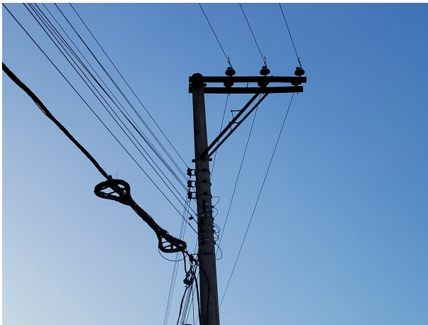
a) An overhead power line.
