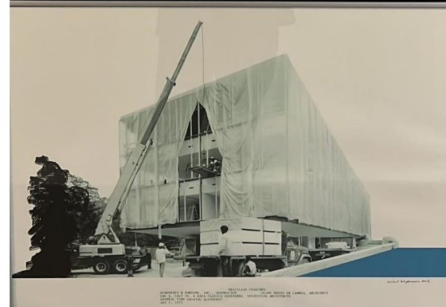
COMPANHIA S. AMARAL, INC. - CONSTRUTORA S. AMARAL 1500 N. W. 10th St. - Miami Beach, Florida - U.S.A. BRASILIAN FRANCHISE - CLAUDE BROSSE DE CAMPA, ARCHITECT 1500 N. W. 10th St. - Miami Beach, Florida - U.S.A. JULY 8, 1970
